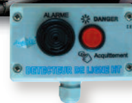
Cabin control monitor outside
